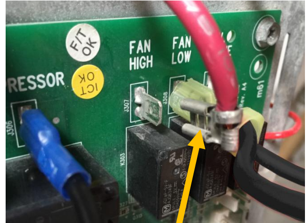
Disconnecting High Speed Fan Cable
