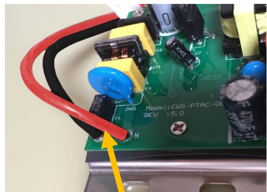
Photo 31. This Red Cable 7 of PTAC-0011 module going to Line 1 of the PTAC system board.
